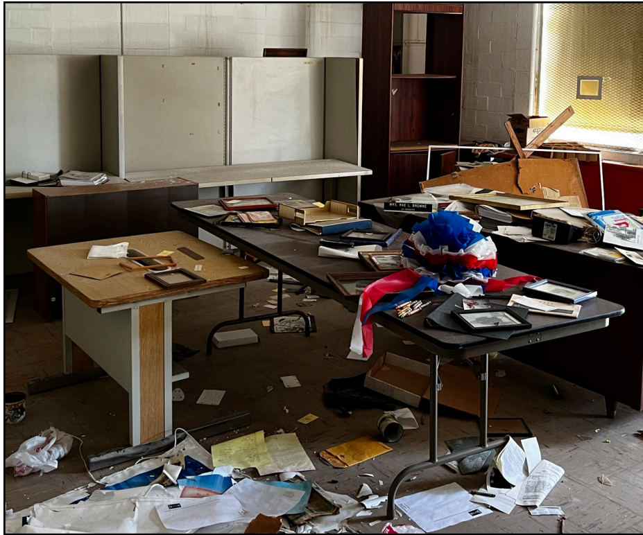
Fig. (013). Instance of vandalism in first level classroom.
