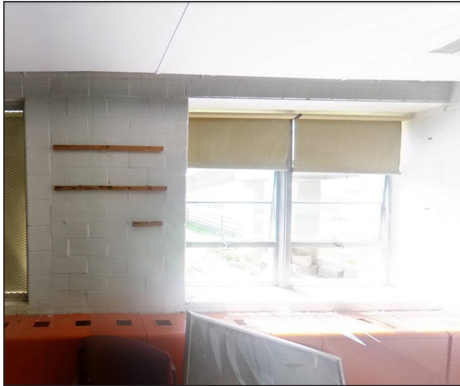
Fig. (009). This broken window on the first level has become a primary access for intruders.
