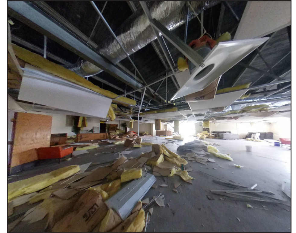
Fig. (011). Destruction to HVAC ductwork on second level.
