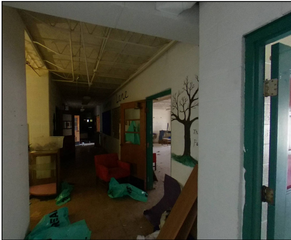
Fig. (014). Hallway full of debris.
