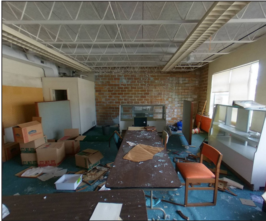
Fig. (007). Instance of vandalism in first level classroom.
