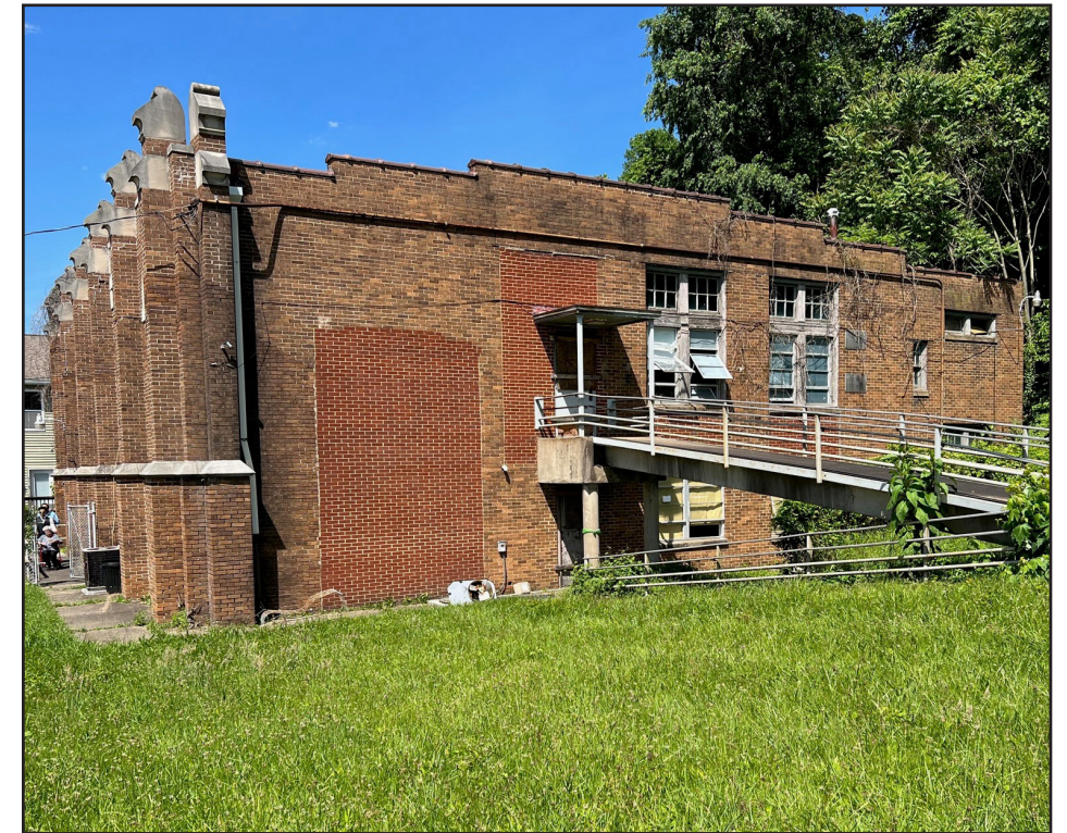
Fig. (018). The south elevation. Notice the overgrown vines on the east side of the building.
