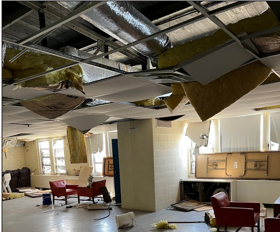
Fig. (010). Destruction of acoustic ceiling tile grid over stage.
