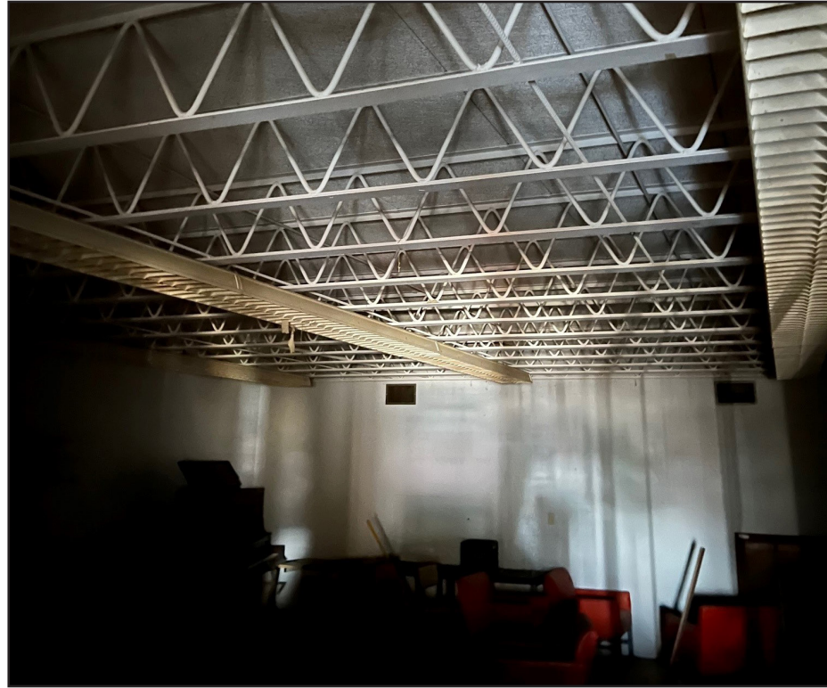
Fig. (015). Existing teachers' lounge ceiling.
